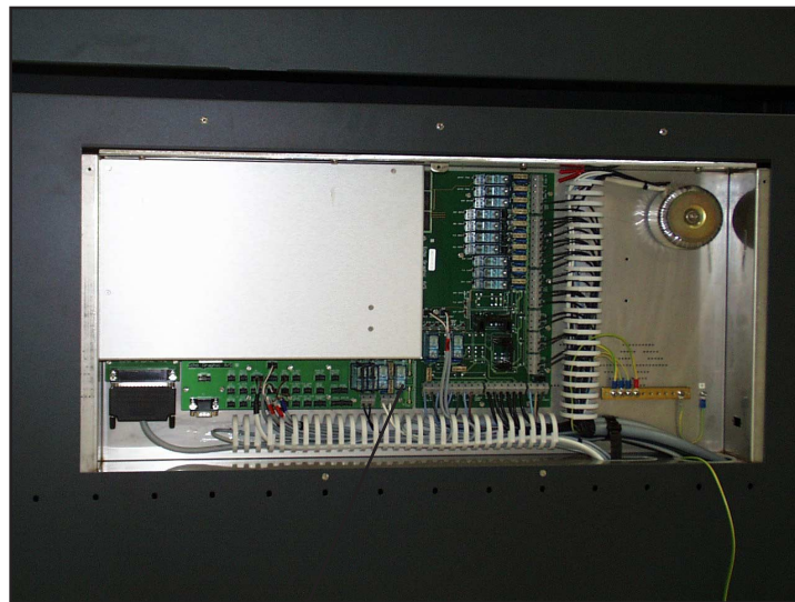
Fig 6-I Low voltage fuses Main power and Conv. motor fuse
